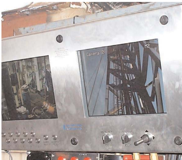
Typical Hazardous Area Dual TFT Screen
